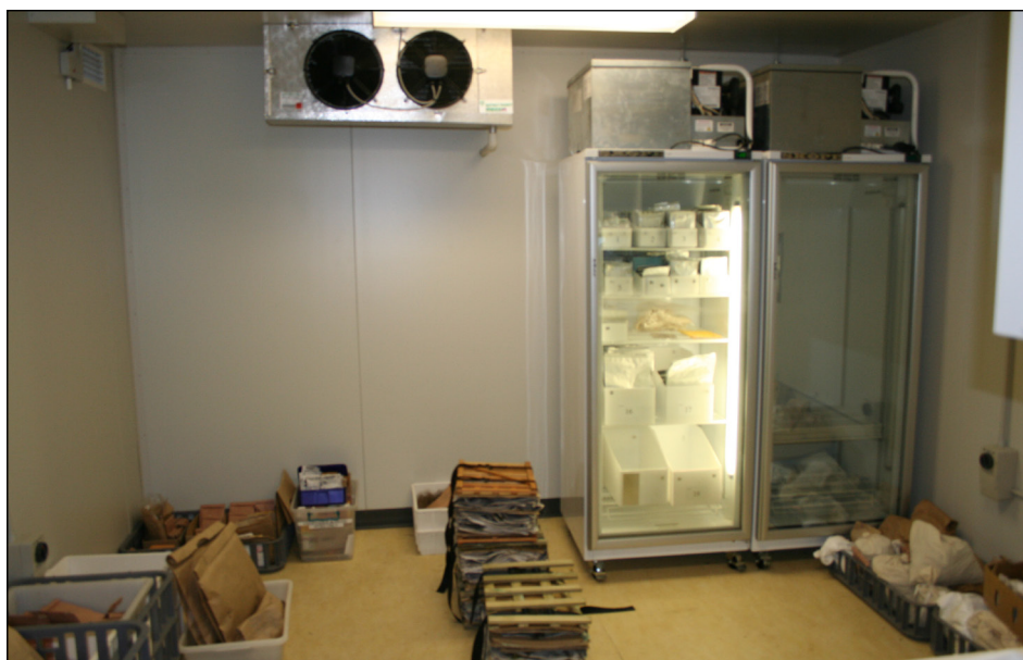
Below: Tasmanian Seed Conservation Centre, Australia - dry room with sorption dryer unit and -20°C chiller cabinets for seed storage
